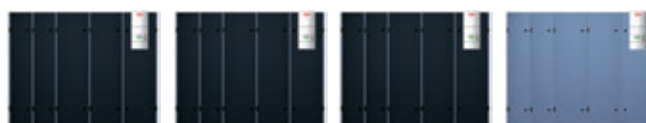
In conventional operating mode, the active A/C units run continuously at full load. The standby unit remains unused.
