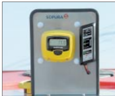
IBC Chemical Metering
