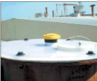
Sulfuric Acid Bulk Storage
