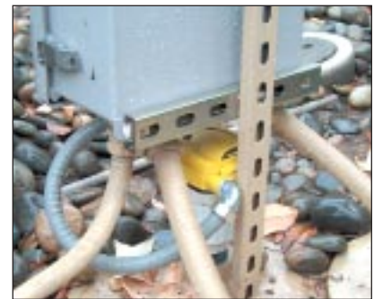
Residential Water Lift Station
