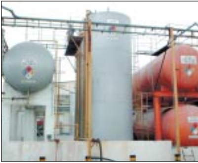
Metal Tank Solutions
