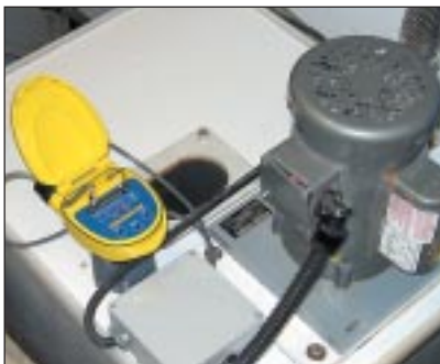
Industrial Waste Lift Station
