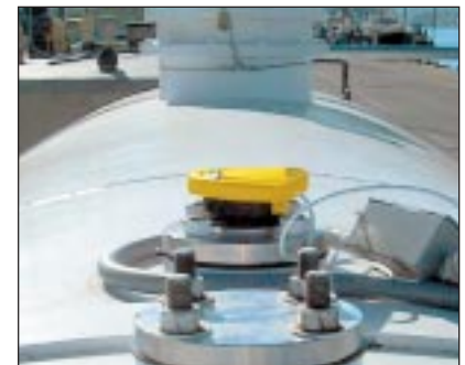
Marine Lube Oil Storage
