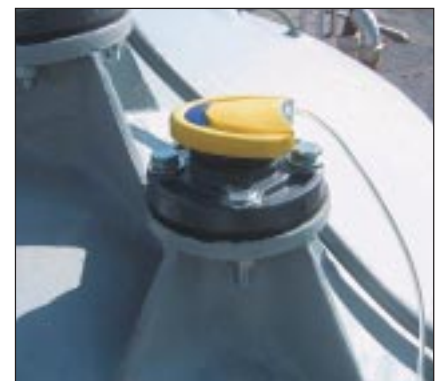
Chemical Bulk Storage
